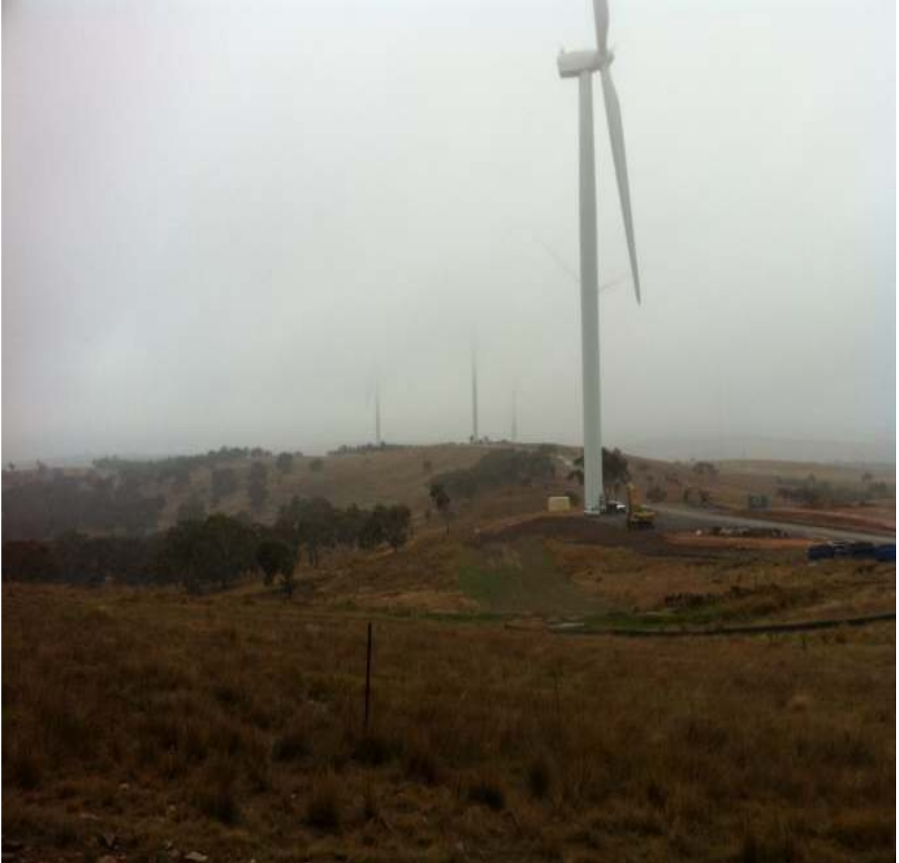
Capital Windfarm 2 – Construction at ‘Woodlawn’ Tarago, Mid 2011. The size of the turbines becomes evident compared to the size of the machinery on the ground. This wind farm is now fully operational.
